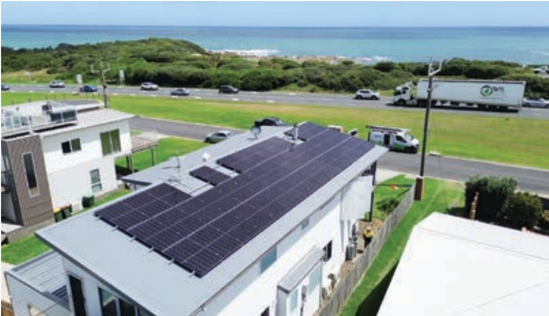
A 15 kW residential solar power system installed by Advanced Solar and Batteries.
