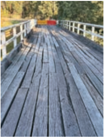
The users of the Stewart Road bridge at Kernot have already sustained significant inconvenience, disruption and cost since its closure early in April and they want to see council seek urgent funding to accelerate the works.
