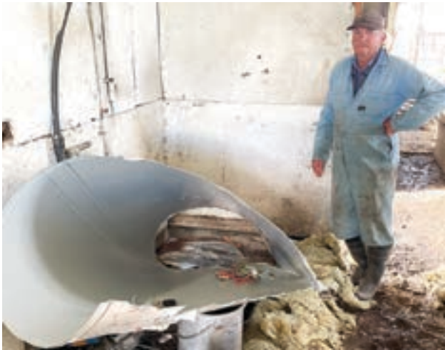
Thieves cut open a hot water service on a farm in Leongatha South to remove all the copper, and Brian and Tony Trotman (pictured) want to warn people about it happening.
