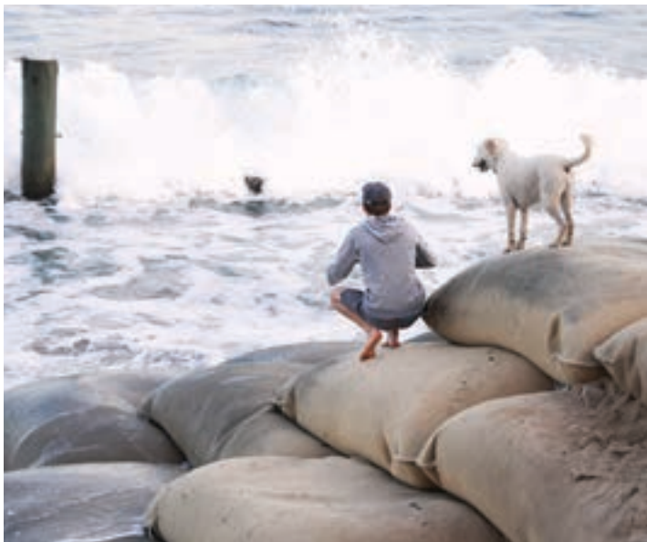
Even on a day of moderate swell last Sunday, waves crashed over the geotextile wall at high tide, also undercutting both ends of the wall as beach erosion marched ever closer to the Inverloch Surf Lifesaving Club.
