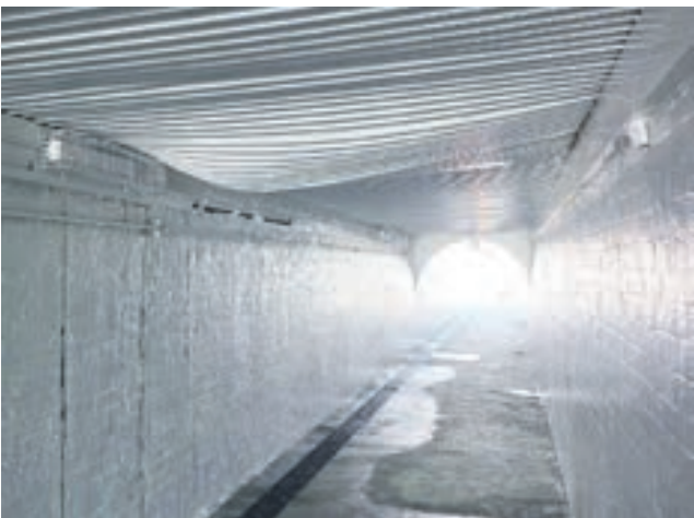
The pedestrian tunnel in Korumburra is closed after the roof caved in.
