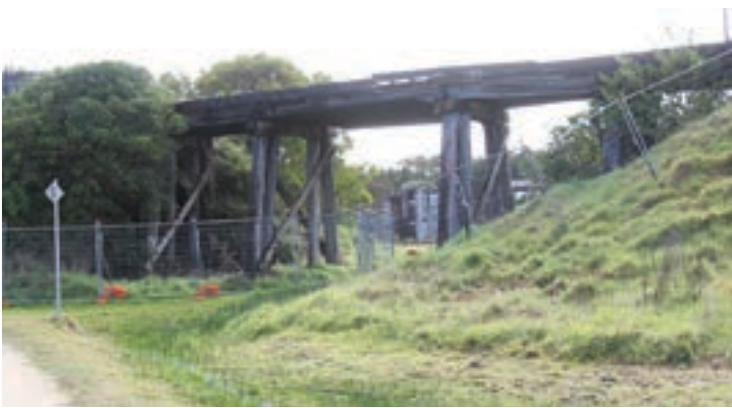
The Kilcunda viaduct rail trail bridge built around 1911 has been out of service for more than 50 years and is now at risk of collapse.
