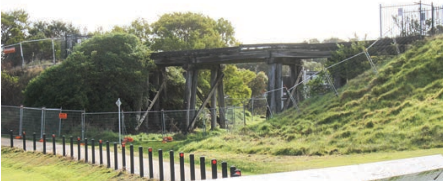
Bass Coast Shire Council has voted to demolish the Kilcunda Viaduct Bridge due to the risk of collapse. B01_2925
