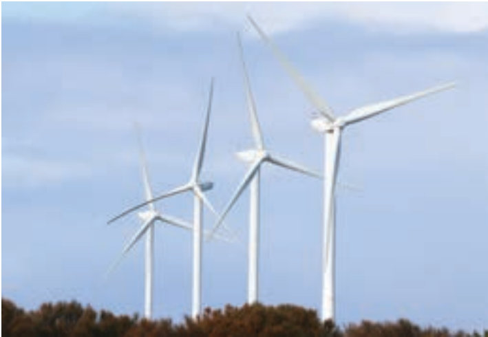
Commissioned in 2005, the six wind turbines at Wonthaggi are now nearing the end of their expected lifespan. W02_3225
