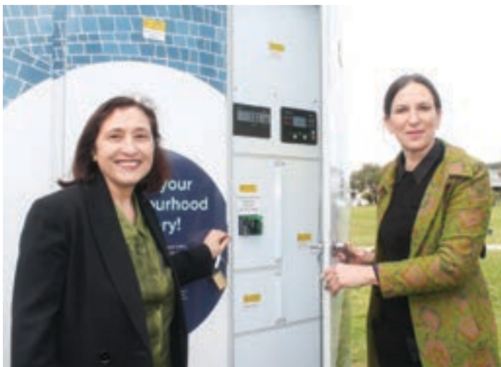
State Minister for Energy and Resources Lily D'Ambrosio MP and Member for Bass Jordan Crugnale MP officially opened six of seven completed neighbourhood-scale batteries on Phillip Island. B29_3425
