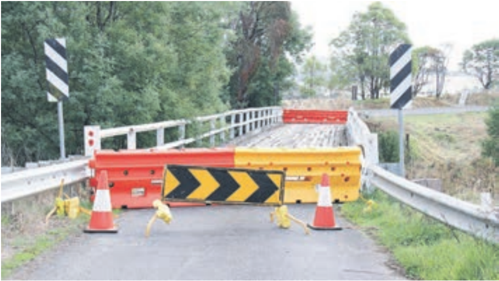
Stewart Road bridge remains closed over the Bass River at Kernot as Bass Coast Council waits on funding. B32_212
