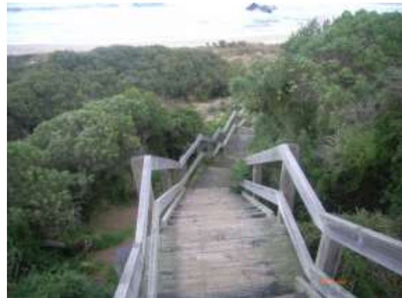
Obs 4 - Although a moderately good timber access point with hazard signage, some areas are slippery and steep, requiring sections to have wire mesh overlays to prevent slipping.
