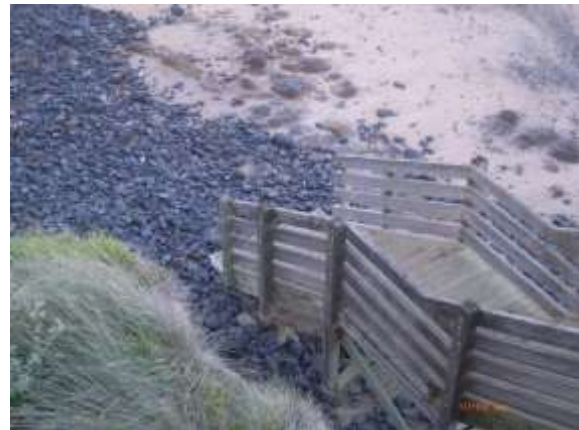
Obs 4 - Stepped boardwalk access directly on loose cobbles stones providing an unstable and uneven walking surface.
