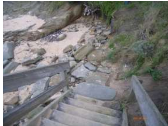
Obs 4 - Stepped boardwalk leads onto an uneven and slippery beach entry surface.
