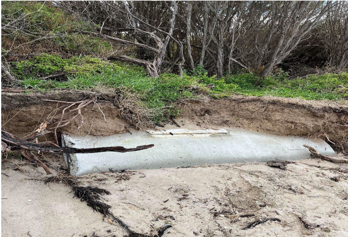
Caption: The exposed septic tanks at Flat Rocks
