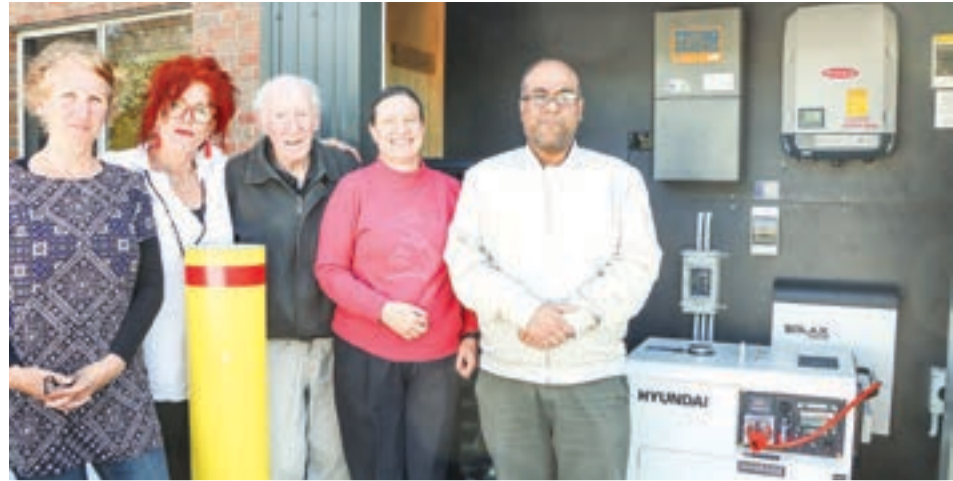
Community Resilience and Reliable Energy Feasibility Study Project Team members Moragh Mackay, Alyson Skinner, Henry O'Clery, Heather Smith and Rakib Shah stand in front of Venus Bay Community Centre's energy resilience equipment. A21_4022
