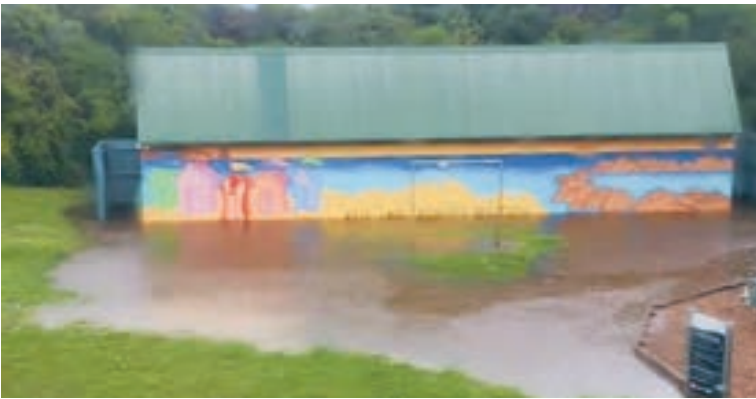
A reported blockage to stormwater outfall pipe at Cape Paterson left the Bay Beach Toilet Block flooded at the weekend but has identified a problem that needs to be addressed.
