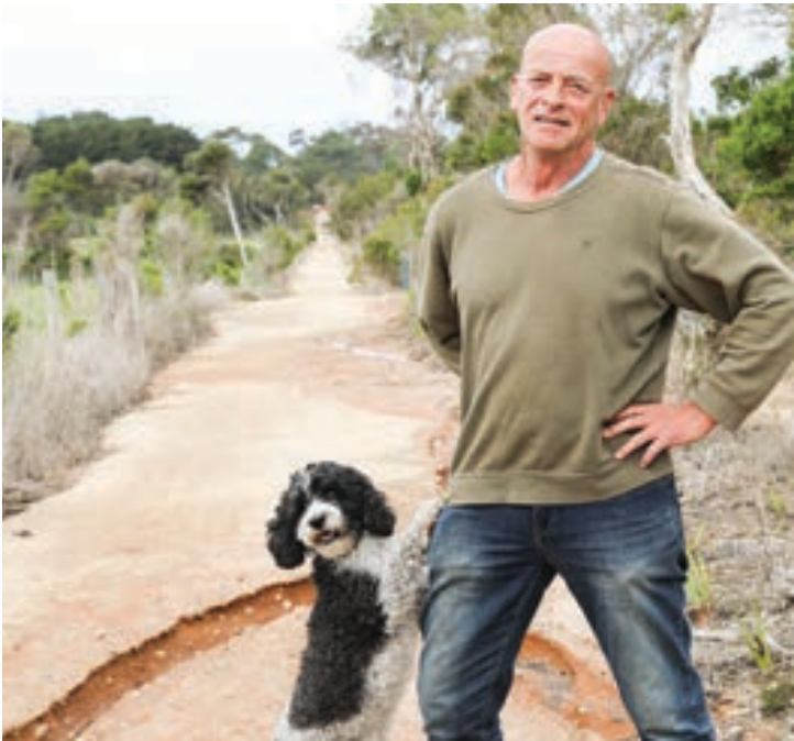
Rod O'Neill from the Inverloch Glamping Company is dismayed by deep washaways on the Wonthaggi to Inverloch shared pathway after recent heavy rain. B26_4625
